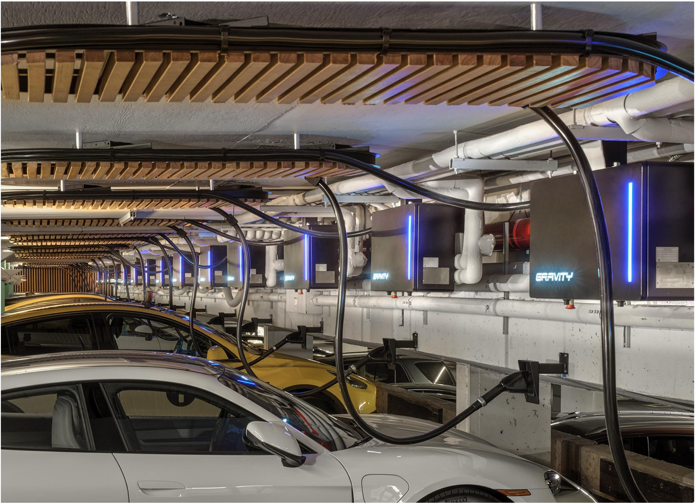
Installation of DEAPs required zero-dedicated space
