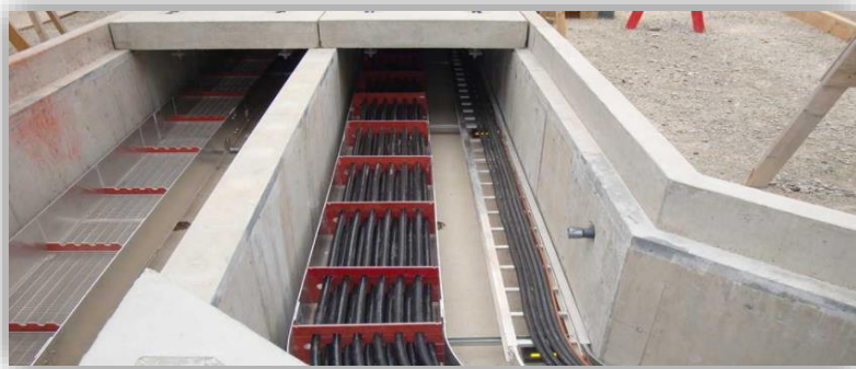
High Voltage/Amperage Underground Vaults = Expensive
