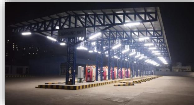
Charging Equipment Protection
