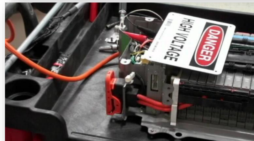
High Voltage Safety Training
